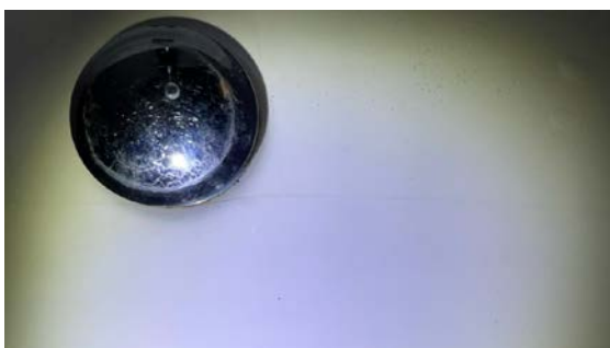
Riss i servant
