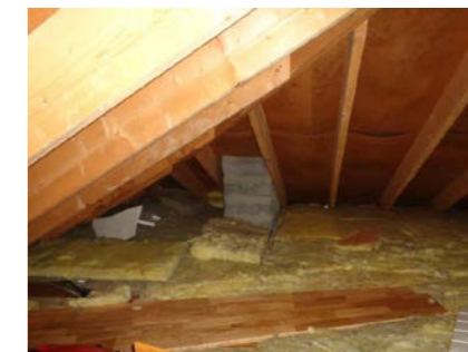
Upusset pipe i knevegg.
