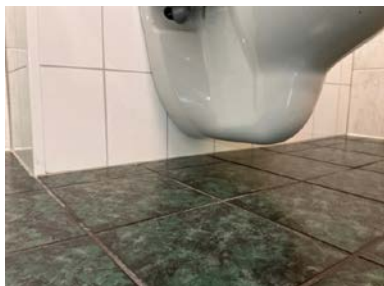
Toalett mangler drenering
