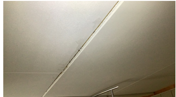
Glippe mellom himlingsplater.
