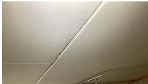
Glippe mellom himlingsplater.
