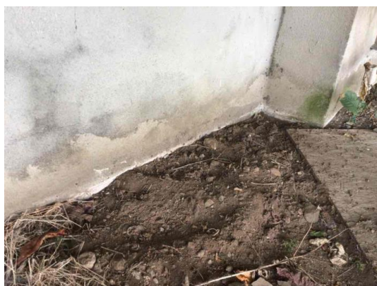
Mangler fuksikring langs mur
