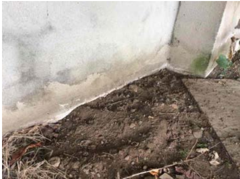
Mangler fuktsikring langs mur
