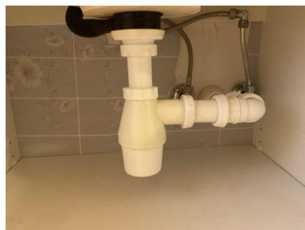
Røropplegg under badervask.
