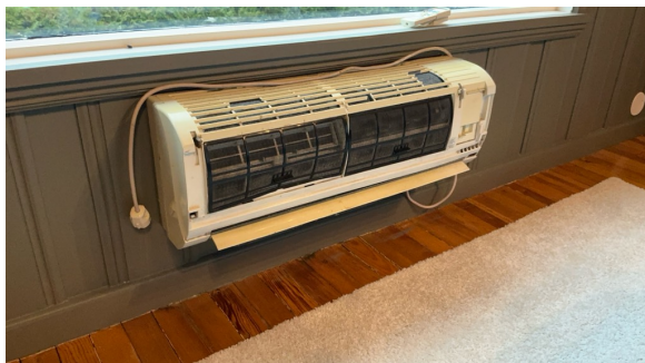
Eldre varmepumpe i stue
