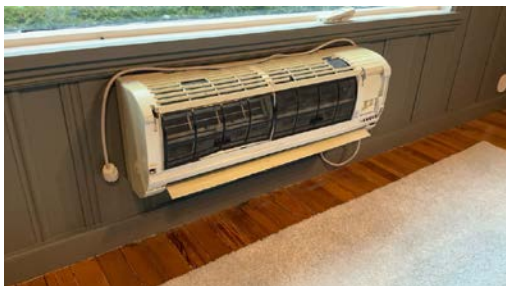
Eldre varmepumpe i stue
