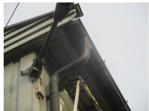
Noe eldre takrenner.
