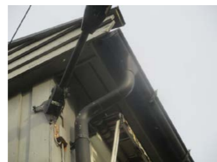
Noe eldre takrenner.
