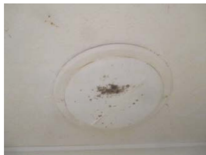
Ventil i himling.
