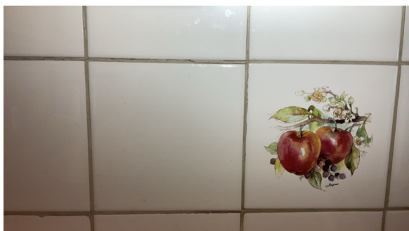
Sprekker i flisfuger
