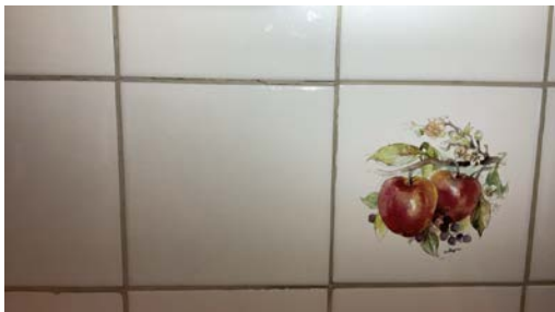
Sprekker i flisfuger
