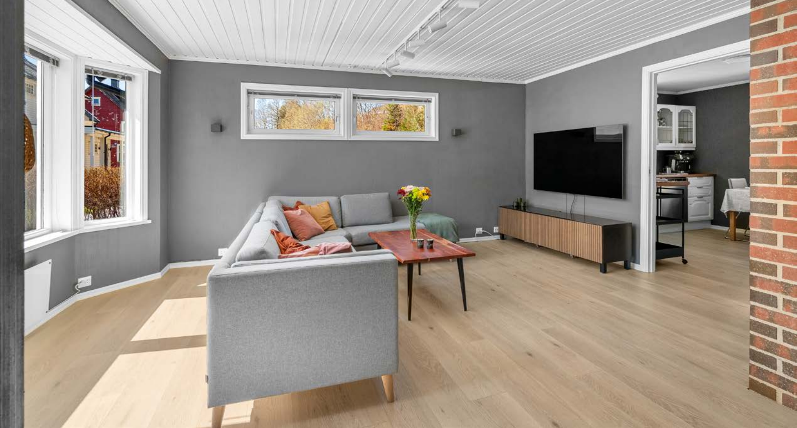
Varmepumpe gir behagelig oppvarming.
