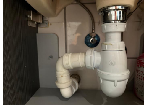
Røropplegg under servant.
