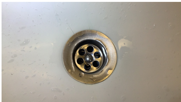
Riss i servant.
