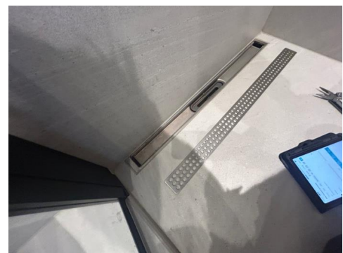
Slukrenne langs vegg
