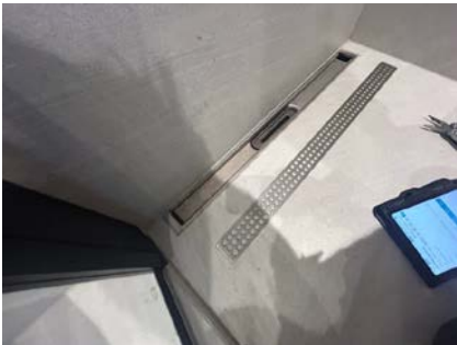
Slukrenne langs vegg
