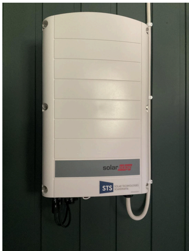
Solcelle inverter i gang
