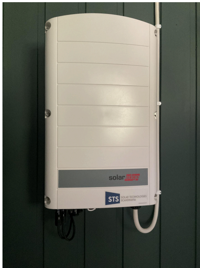
Solcelle inverter i gang
