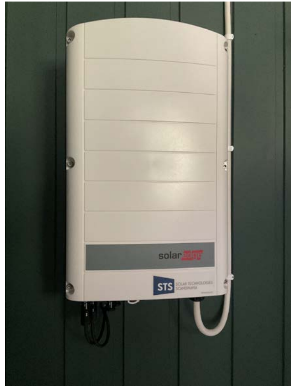
Solcelle inverter i gang
