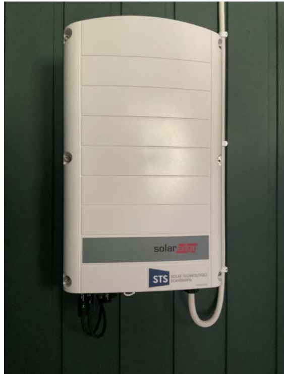
Solcelle inverter i gang
