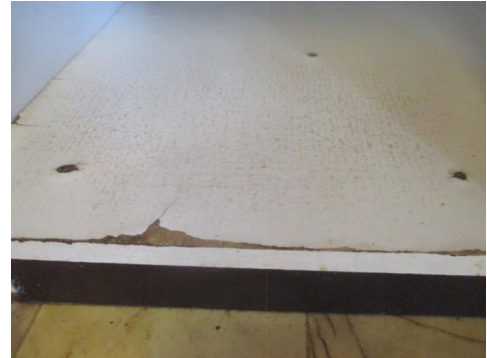
Eldre fuktskader under vask.
