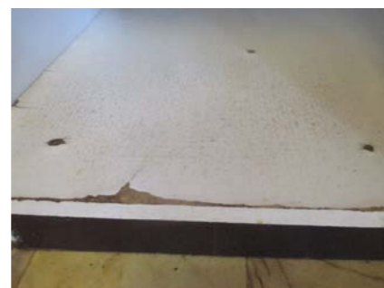
Eldre fuktskader under vask.
