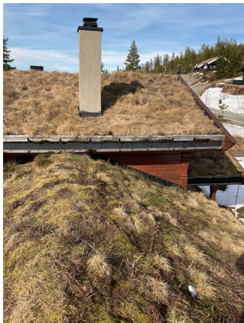
Manglende adkomst for feier.
