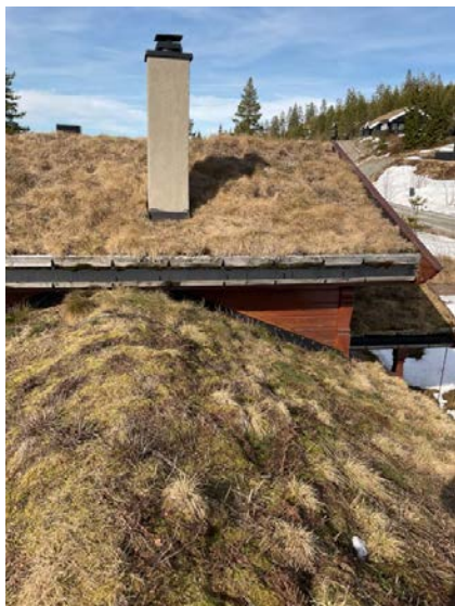
Manglende adkomst for feier.
