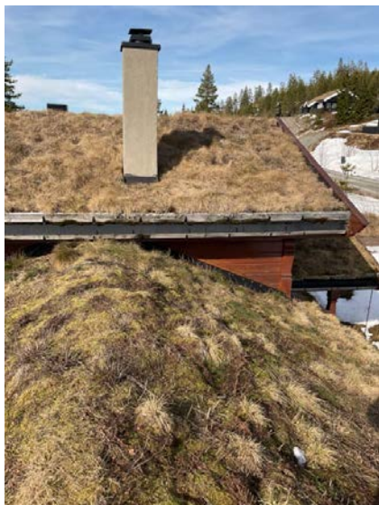
Manglende adkomst for feier.
