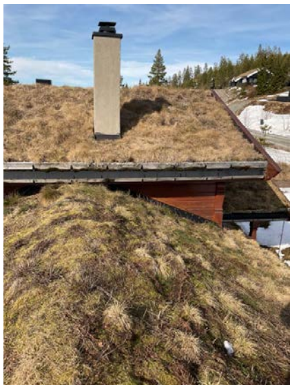
Manglende adkomst for feier.
