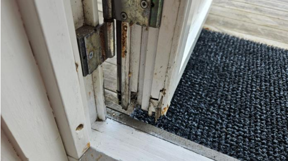
Fuktsvell i karm.
