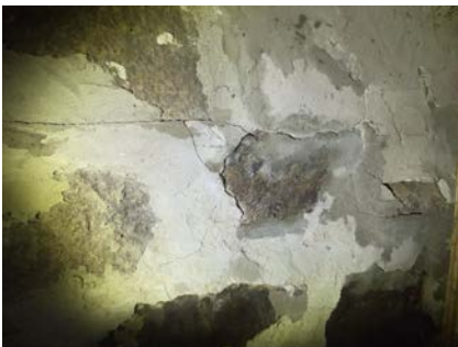
Sprekker gammel natrusteinsmur
