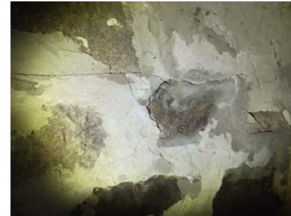
Sprekker gammel natrusteinsmur
