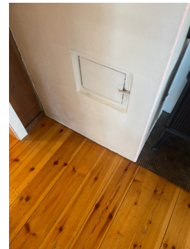
Ildfast plate mangler under sotluke.
