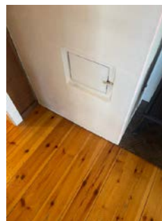
Ildfast plate mangler under sotluke.
