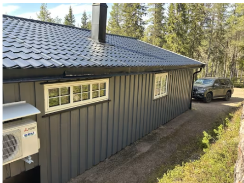
Manglende adkomst for feier.
