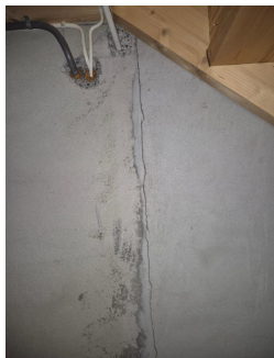
Sprekk i vegg i kott under trapp.
