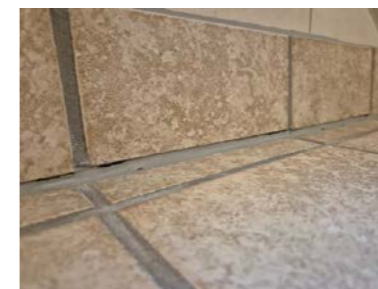
Sprekker i mykfuger.
