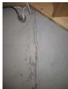
Sprekk i vegg i kott under trapp.
