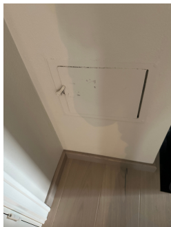
Manglende ildfast plate under feieluke
