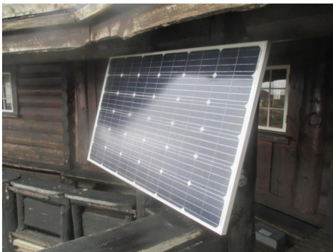
Noe eldre solcellepanel.
