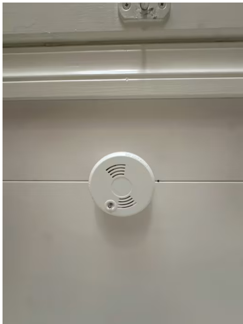
Viser brannmelder montert i himling.
