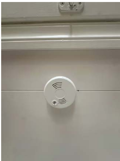
Viser brannmelder montert i himling.
