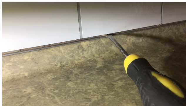
Mangler fuging i underkant
