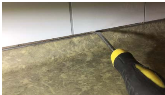
Mangler fugging i underkant
