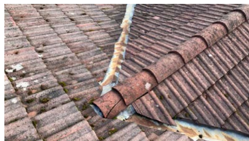
Rust i gradrenner.
