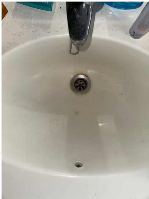
Krakelering i servant.
