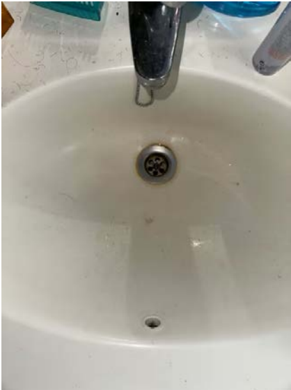
Krakelering i servant.
