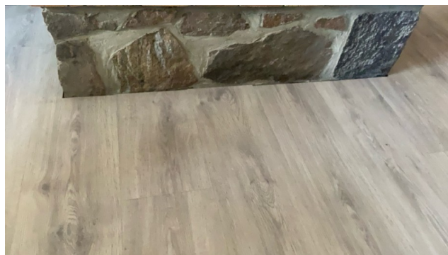
Ildfast plate mangler under/foran ildsted.
