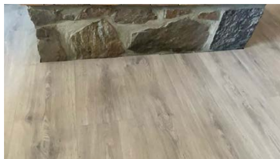
Ildfast plate mangler under/foran ildsted.
