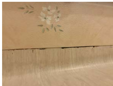
Overgang tapet/ gulvbelegg
