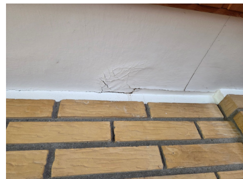
Eldre fuktskade i himling
