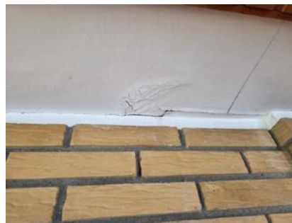
Eldre fuktskade i himling
