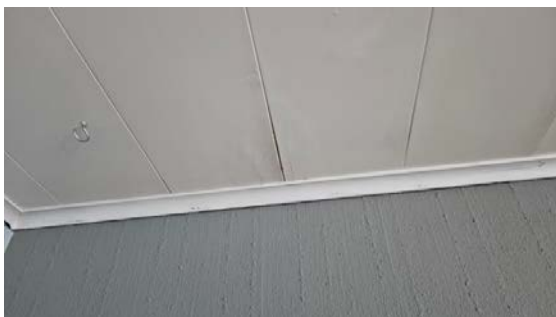
Fuktsvell i himling i stuen.
